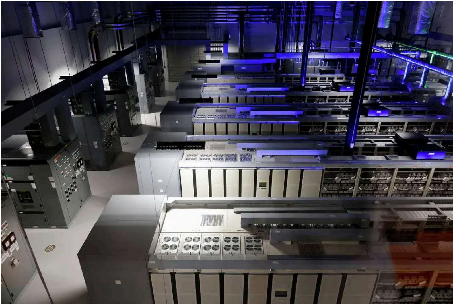
An overhead view of the Dallas TX1 electrical plant at the NTT Data center in Garland, Texas, June 23, 2025. Tom Fox/TNS
