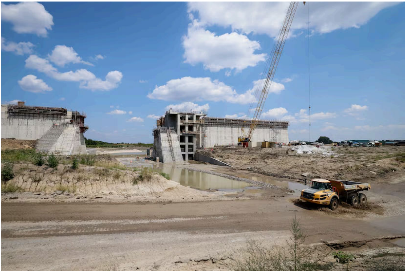
A dump truck drives through a channel redirecting the North Sulphur River to pass between the unfinished spillway at the future Lake Ralph Hall on Aug. 7, 2025, in Fannin County. Once the dam is complete, the spillway will release overflow water back into the higher than the underground pipes that will utilizing gravity to supply a nearby pump station with water. xpand access and preserve the essential resource North Tex
