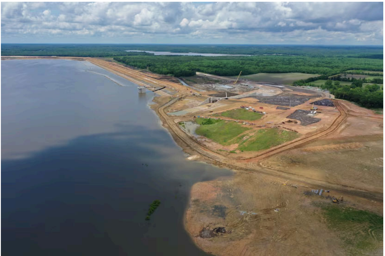
Bois d'Arc Lake is filling quickly and as expected, North Texas Municipal Water District said. Construction of the lake's dam and surrounding offices are taking place and the lake is planned to begin operating as a reservoir in 2022.
