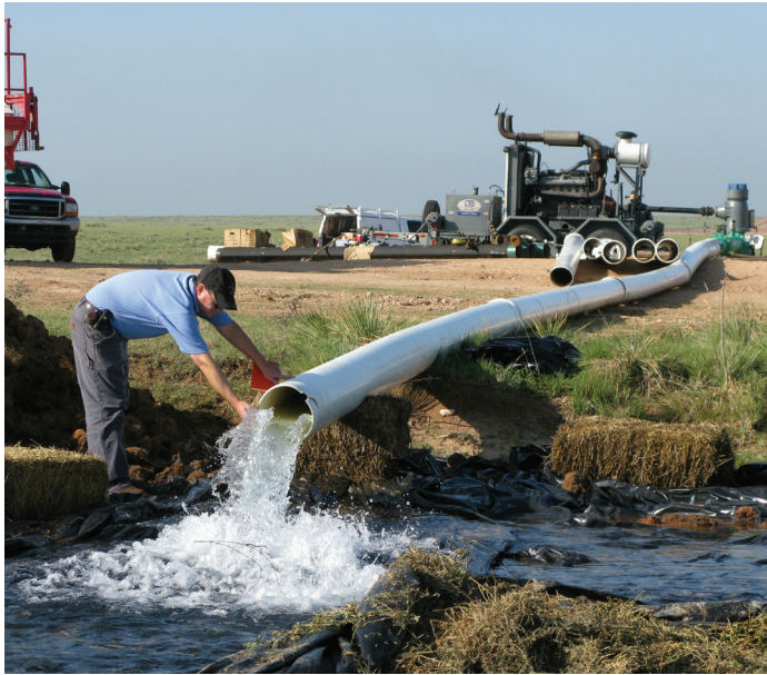
Prototype supply wells demonstrated production capacities ranging from 850 to 1,140 gallons per minute.
